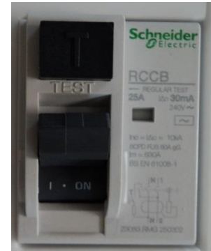
Figure 9: RCCB for the workstation
