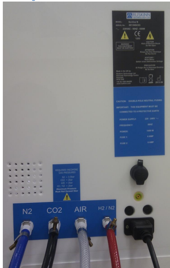
Figure 3: Gas and electrical connections
